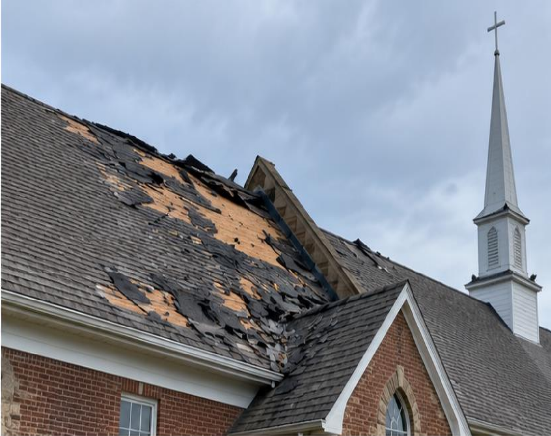
WIND: missing/lifted shingles, exposed decking
